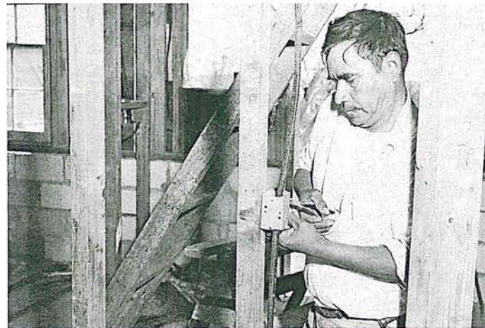
Johnny Valdez, installing an electric outlet in a self-help home, Meadow Wood, Texas, a joint OEO-Farmers Home Project.
