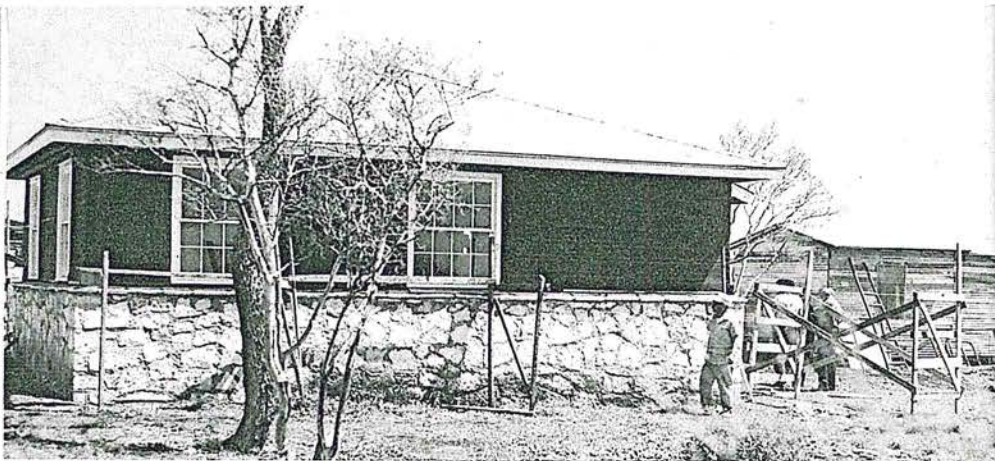
The new home of Mr. Jose Vasquez is ready for stucco. Meadow Wood, Texas.
