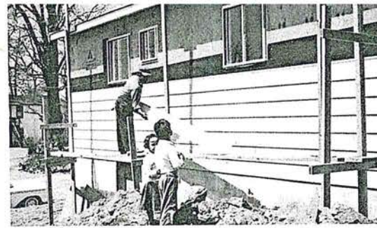
Reyes family self-help house with father putting up siding. Chester County, Pa. This father of 9 children, working for $1.00 per hour was offered $3.25 an hour as a construction worker, utilizing the skills he had shown in the self-help building project. He had to decline the better job because he lived in a house owned by his employer and no other landlord would rent him a house because of the number of children.
