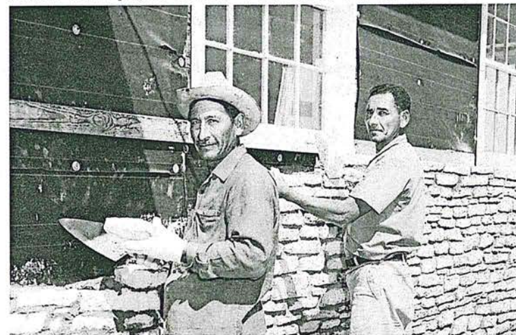
Jose Torries and Frederico Gutierrez working on self-help housing, OEO/Farmers Home project, Meadow Wood Acres, near San Antonio, Texas.
